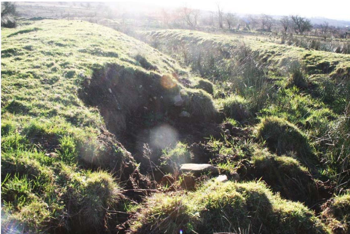
Figure 11.11 – Erosion to the bank at the south-west, looking south.
