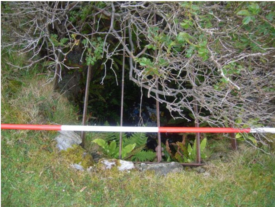
Figure 2.11 - Metal grill covering furnace shaft at Murlough Bay lime kiln (from Welsh 2001, figure 16).
